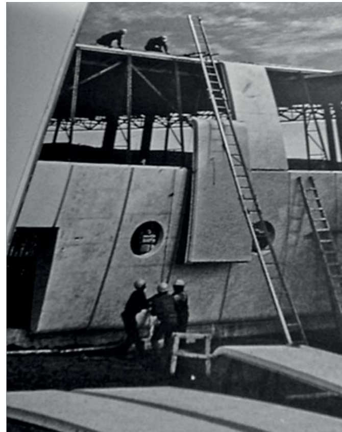
FIG. 12. ASSEMBLING OF PREFABRICATED PANELS FOR THE GORDON ROBERTSON EDUCATION CENTRE. | REPRODUCED FROM PGL ARCHITECT, ARCHITECTURE DE PGL 1959-1975, MONTRÉAL, 1975 (N.P.).
